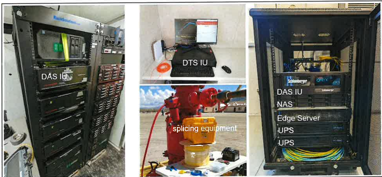
Figure 7: Fiber optic interrogator equipment.
